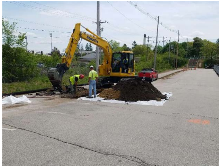
Fig10: McCourt continue to remove pavement and dig test pits in A lot. Viewing southeast.
