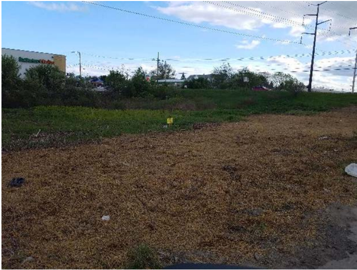
Fig 5: Straw broadcasted over exposed soil area between Strs. F107-136 and 137. Viewing south.
